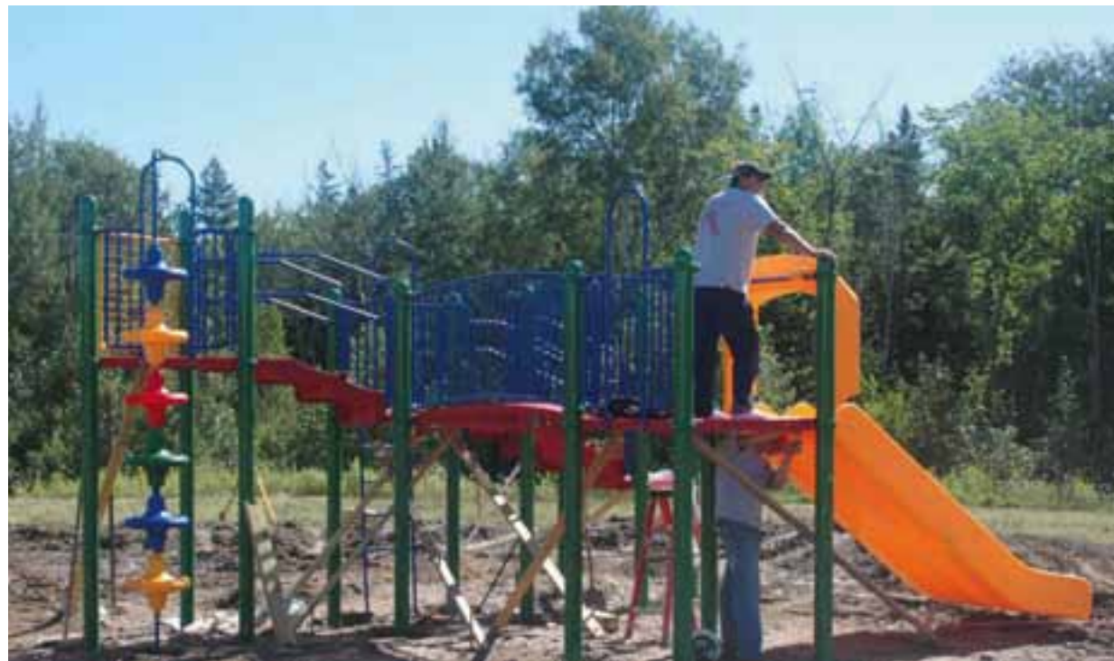
Above, part of the crew of Saf-Play Services erecting the new playground equipment at the Chi Mukwa Community Recreation Center during the last week of August. Below, Sydney White of Sault Ste. Marie initiates the new gear on the day of the official grand opening.
