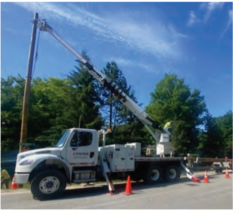
Hessel Caution Light Project — Installation located at the intersection of 3 Mile Rd. and Nopaming Drive, Hessel, Mich.
